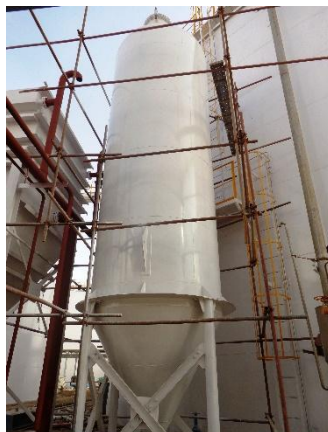
Degassing Tank for Biogas Plant
