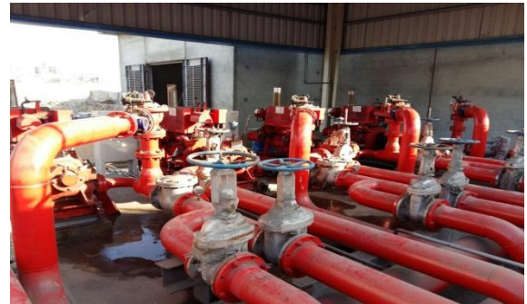
Interconnecting Plant Piping
