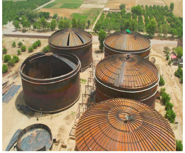
Biogas Digester Tanks
