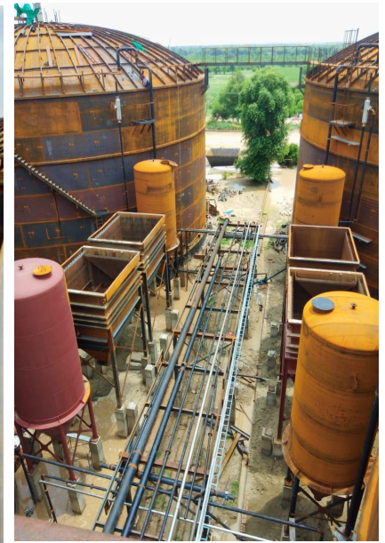
Degassing Tanks, Lamellar Separators
