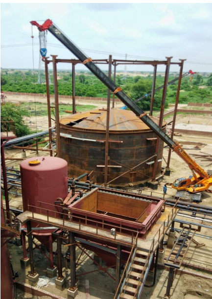
Gas Holder Tank
