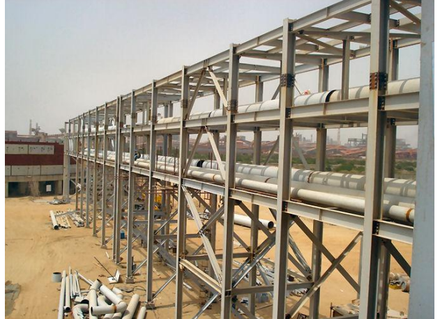
DRI Pipe Racking
